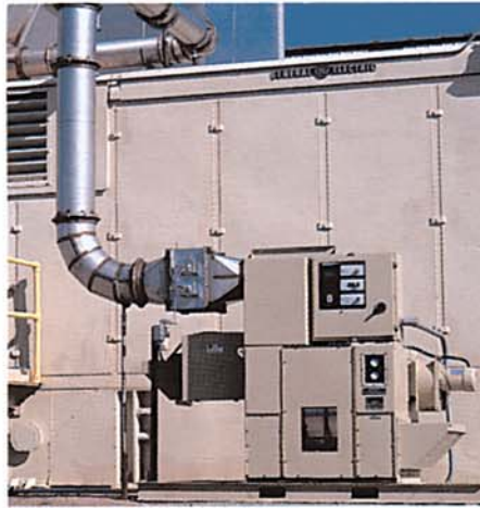
The Munters dehumidifier is weather tight so it was installed outdoors at low cost.
