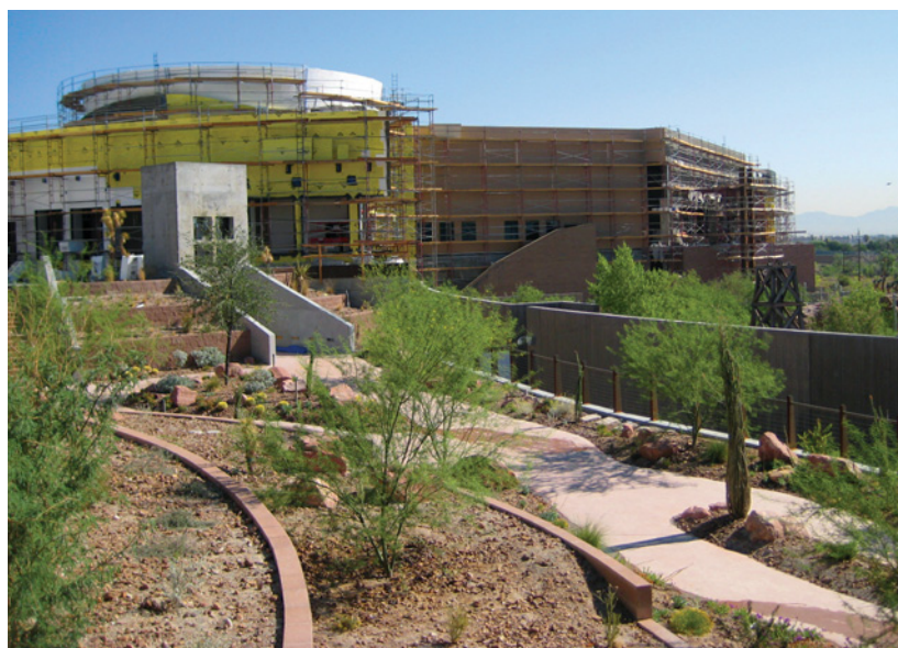
The Springs Preserve in Las Vegas, Nevada has selected the OASIS indirect/direct evaporative A/C system as part of their sustainable building efforts.
